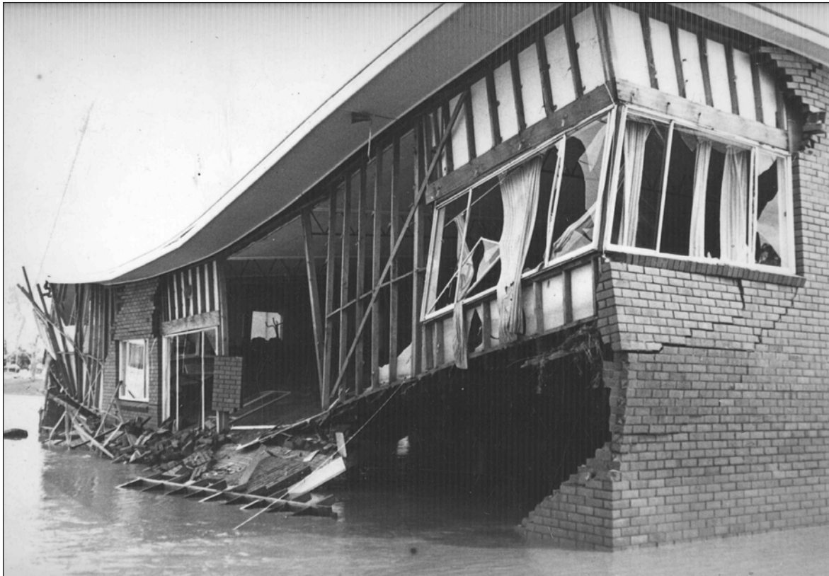
Figure 2 Severe structural damage to buildings of traditional design and construction
