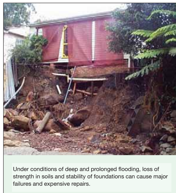
Figure 42 Undercutting from erosion
