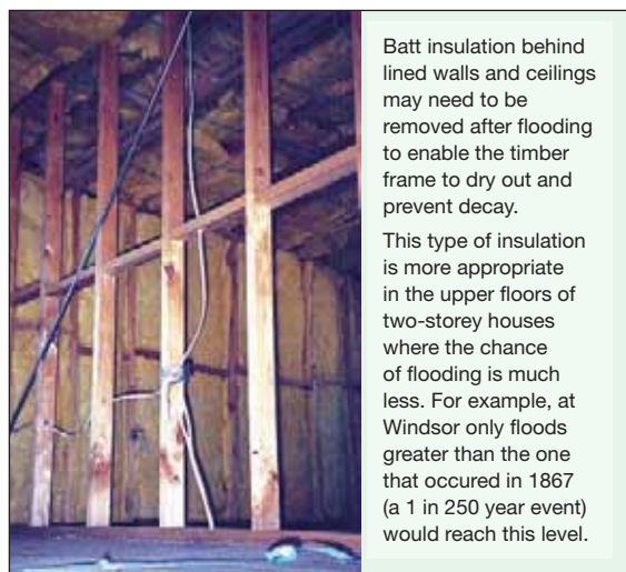
Figure 96 Problems with batt insulation
