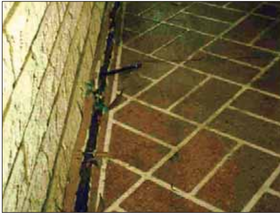
Figure 120 Brick wall bowed inwards due to water force
