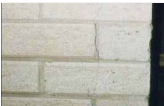
Figure 121 Vertical cracking at corner due to bowing of adjacent wall
