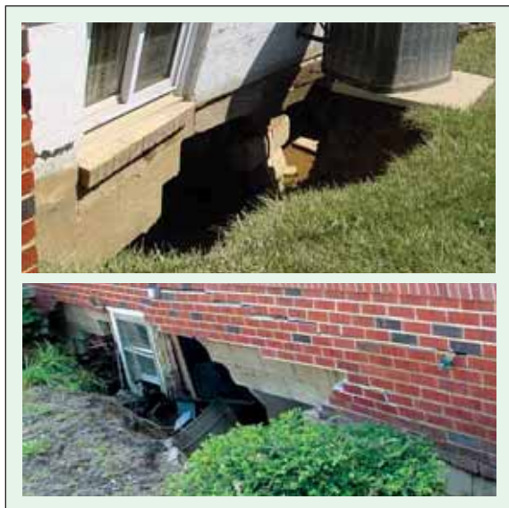
Figure 16 Collapse of walls due to hydrostatic pressure
